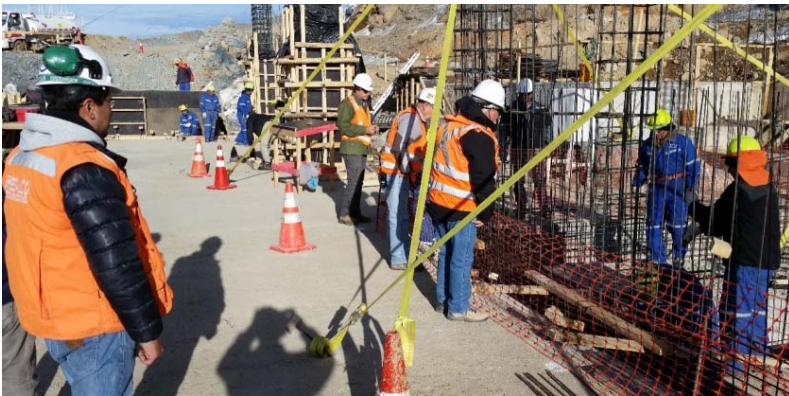
Construction site managers supervise the safe placing of rebar for the summit facility foundation columns on the Cerro Pachón site. Managers wear orange or red vests with white hard hats; workers wear blue overalls and yellow hard hats. Note that housekeeping is excellent on the construction site.
